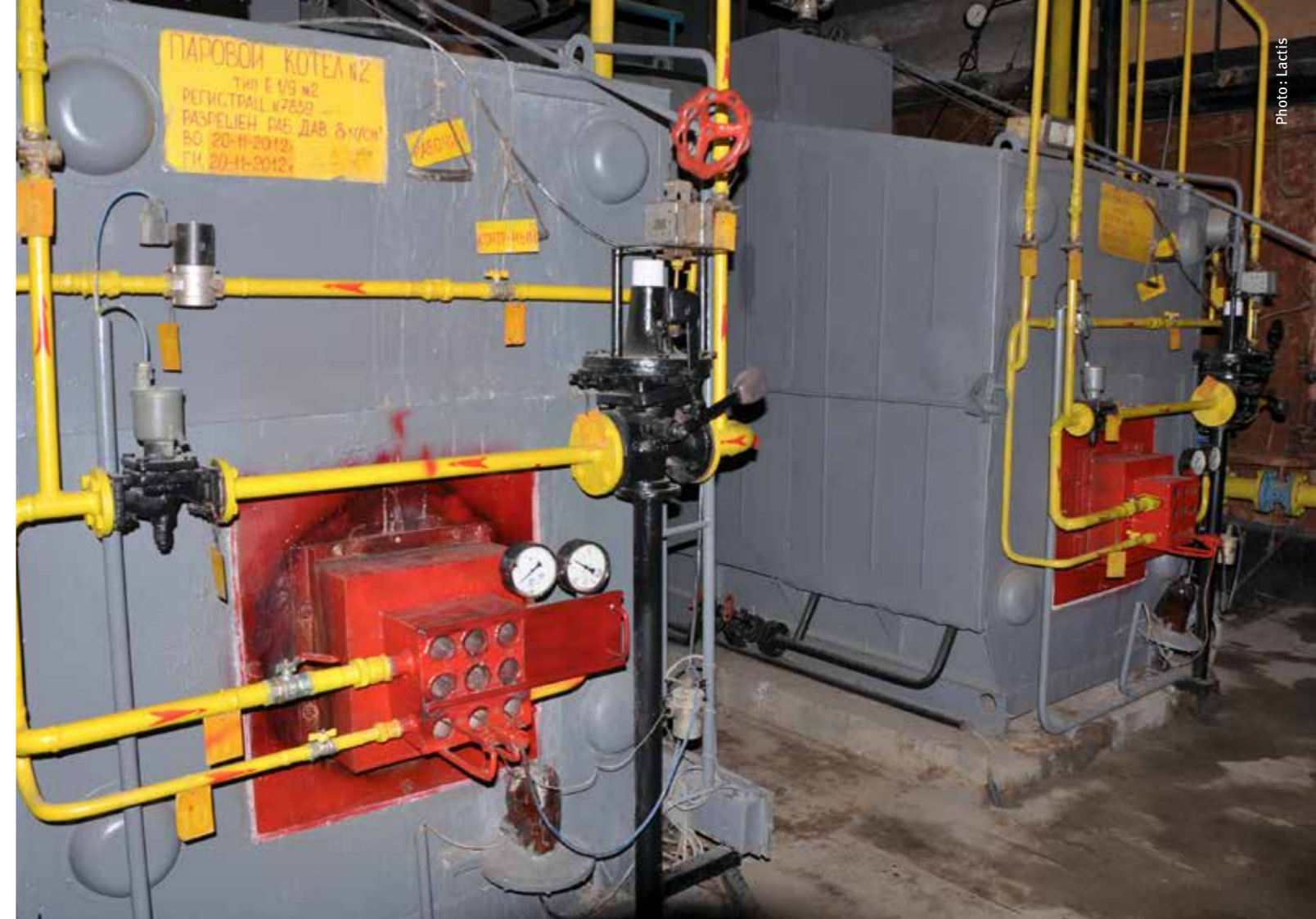
The air intake for the boilers was optimized by installing manual closers, leading to one boiler being switched off completely.
